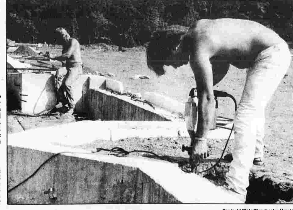
HARD AT WORK — Stanley Baldyga of Ellington, left, and Paul Lenares of East Windsor, put some finishing touches on the concrete with jackhammers for the new post office on Sheldon Road. Both work for NAEK General Construction of Vernon.
